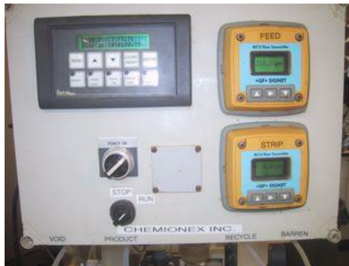
Figure 3: IX Pilot Plant Control Panel
